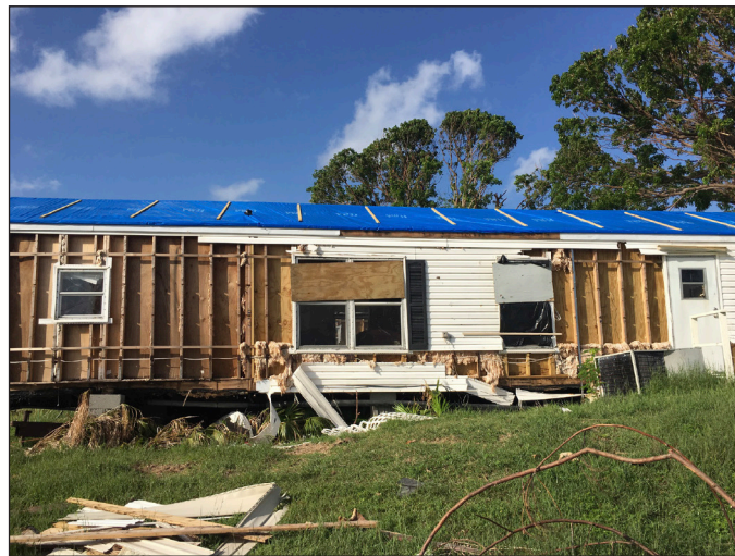
After Hurricanes Irma and Maria in 2017, inspection teams reported many manufactured homes experienced near-total damage cause by high winds.
