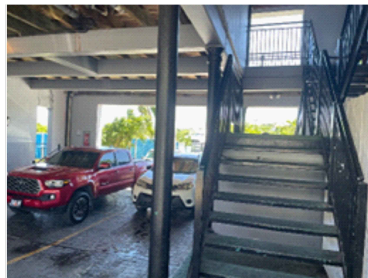
PHOTO 06: INTERIOR VIEW OF CENTRAL OPEN AREA LOOKING SOUTH ON 1ST FLOOR FOR PROPOSED MODIFICATIONS - BUILDING A
