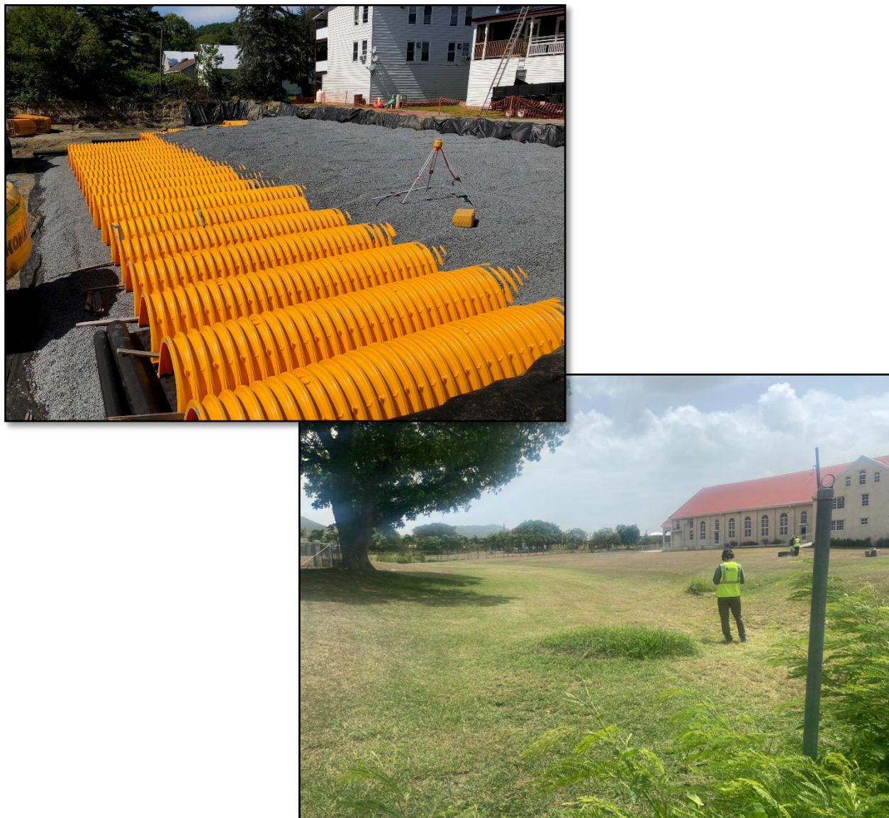
Figure 77. Example photo of subsurface infiltration chambers (above) and major gut channel near the Bethel 7th day Adventist Church (below).
