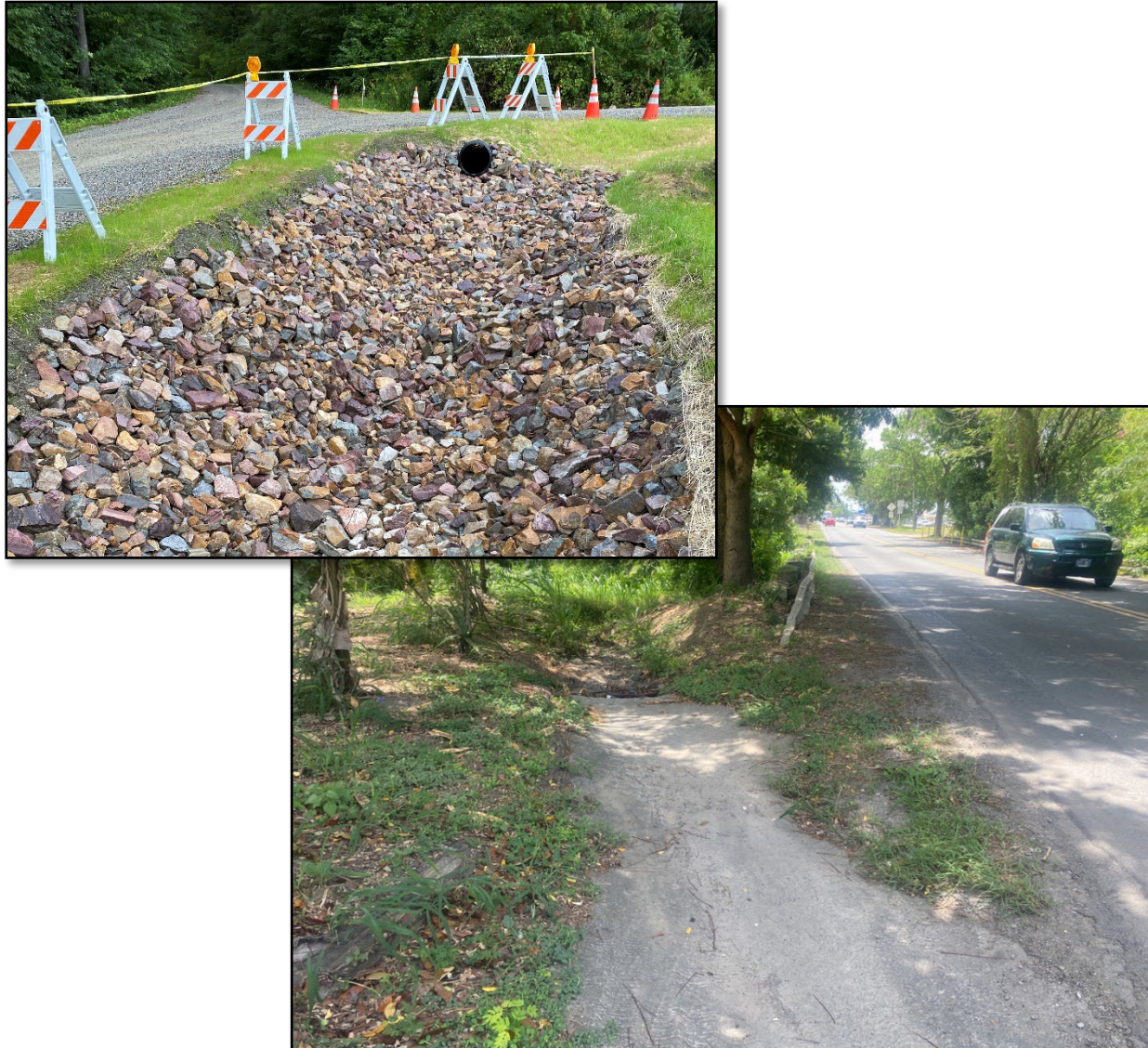
Figure 79. Example photo of stabilized channel with stone (above) and existing site conditions on Centerline Road. (below).
