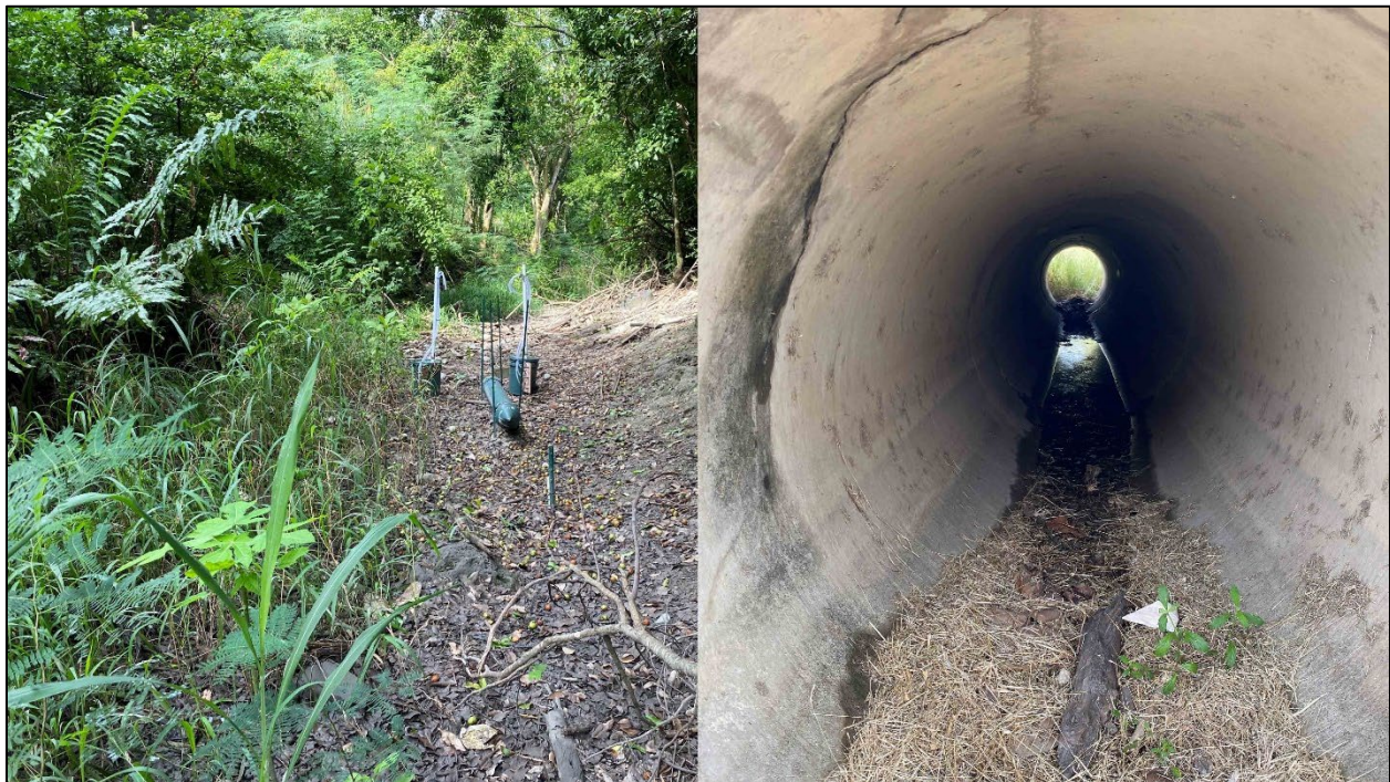
Figure 55. An Onset HOBO U20 Water Level Logger at gauge station SRB01 (left). Water flowing through a concrete structure (right).
