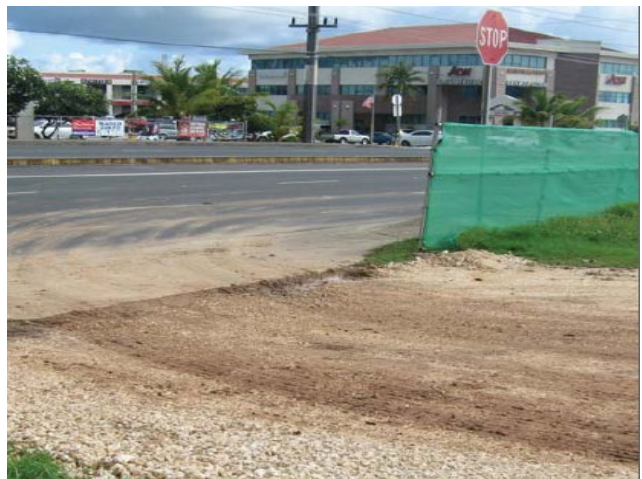
Sediment tracking onto road and buildup shows that this entrance has not been maintained (Guam EPA).
