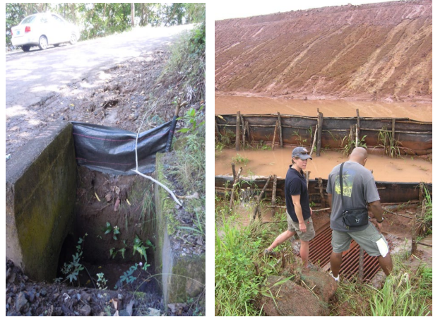
(Left) Silt fences are not effective in ditches. (Right) Use multiple rows of fencing if needed for large drainage areas or to add a level of needed protection.
