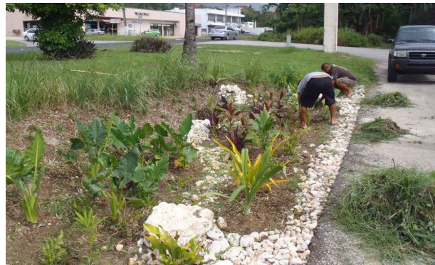
Maintenance activities for vegetated filters include: watering after installation until plants are fully established and weeding, particularly during the first year.
