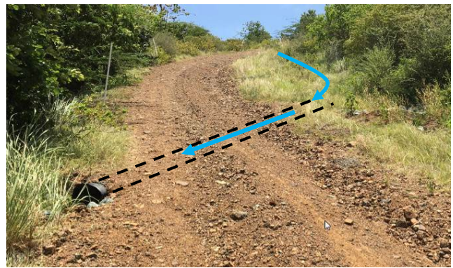
Underground pipe used to convey ditch flow to the opposite side of the road.
