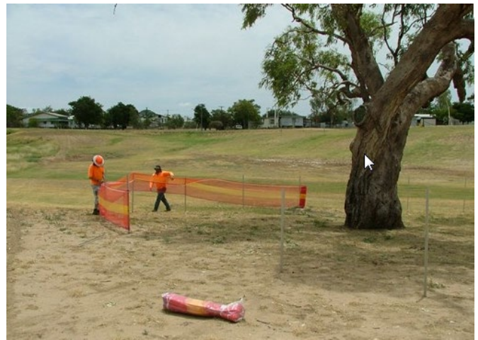
Bright orange construction fencing used for tree protection should be protective of trunk and roots.
