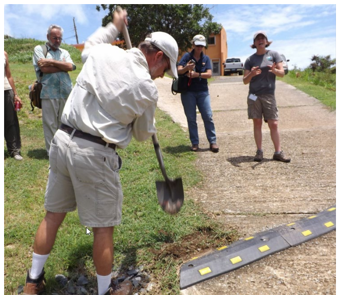
Small maintenance actions like removing buildup at the inlet point may be the one thing needed to keep a practice operational.
