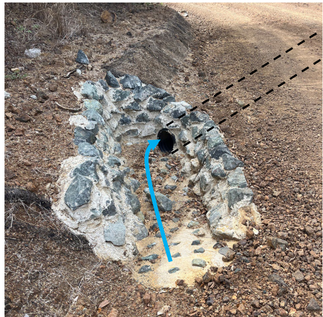
Grouted rock headwall around this cross-drain inlet serves as a ditch block and stabilizes inlet point.
