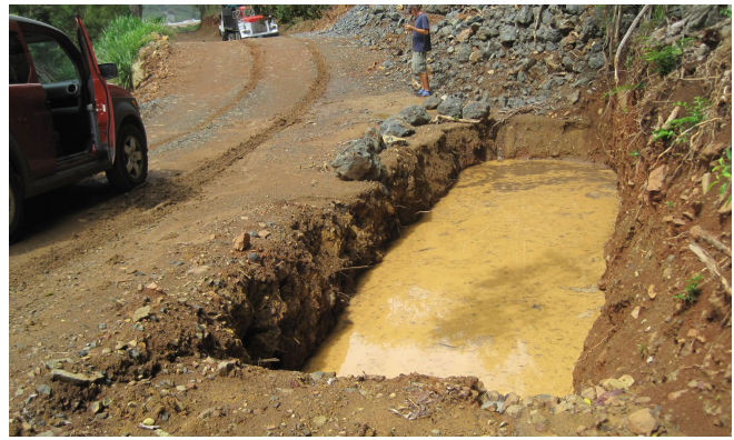
A sediment trap collects runoff from a construction site on St. Thomas East End.
