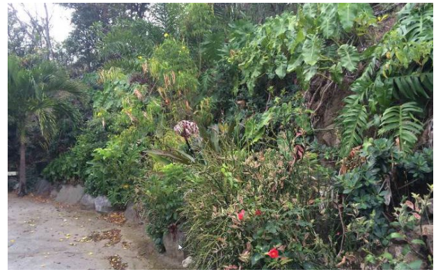
This cut slope on a residential driveway in the BVI was stabilized with stone walls and landscape vegetation—a win/win for the homeowner and downstream coral reefs!
