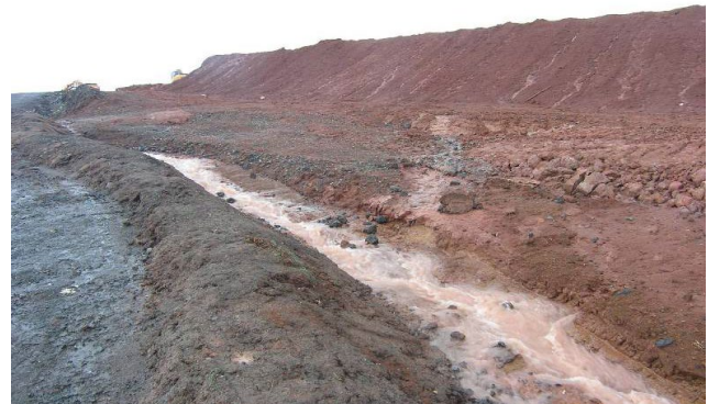
This ditch is carrying high velocity runoff through an exposed construction site. The channel should be stabilized and have check dams to slow runoff and prevent erosion.
