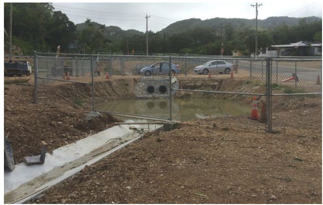
Residence time is too short for this pond to be effective, as evident by the short distance between the inlet as outlet as well as the relatively low outlet invert elevation.
