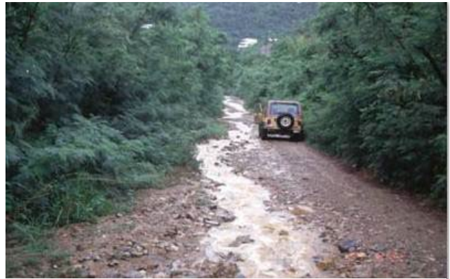
Runoff conveyed down the travel lane will quickly concentrate and erode surface materials. Better drainage designs aim to get water off the road surface at multiple intervals. The length of flow on this road shows an extended and undesirable surface travel time (photo: Coral Bay Community Council).
