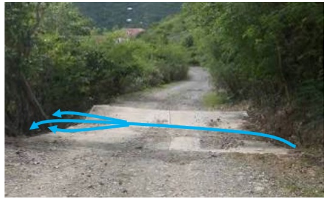
Broad-based dips carry concentrated flows from road surface, ditches, or guts to a stabilized outlet.
