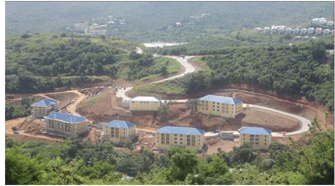
The extent of exposed soils at this steep-sloped construction site on St. Thomas illustrates why proper use of ESC measures is important for protecting downstream resources.
