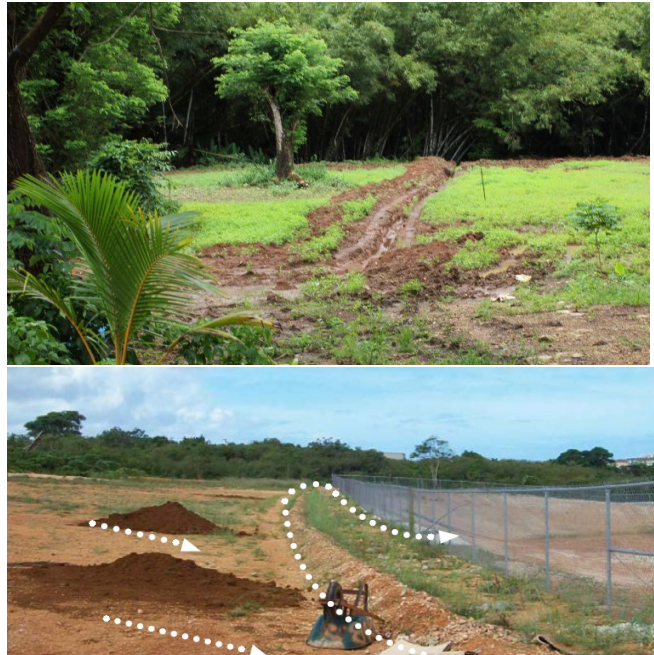
(Top) Diversion swale used to convey off site flows away from construction activity. (Bottom) Berm constructed at the perimeter of sediment basin to convey flows to a stabilized inlet into the basin (Guam EPA). White arrows indicate intended flow paths.
