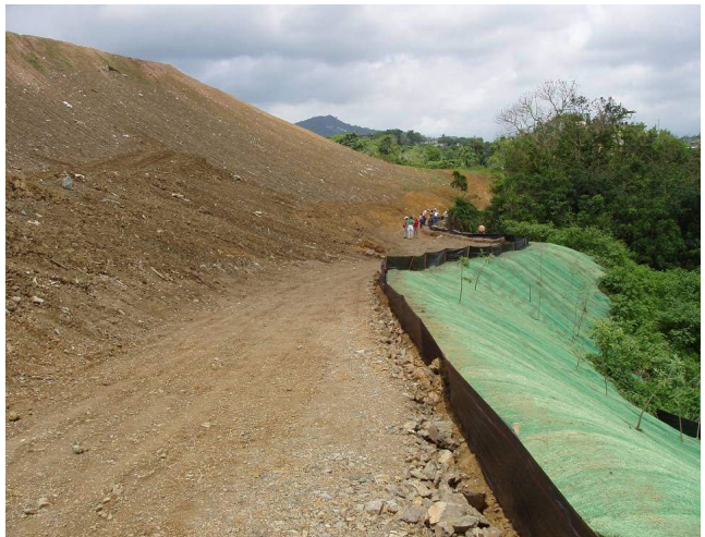
(Top) Installation of straw filled ECB lengthwise down a side slope. (Bottom) Example of a stabilized and unstabilized slope. Lower slope has erosion control blankets with green plastic mesh to protect steep slopes while vegetation becomes established. Think carefully about using plastic as it is not ideal for animals and is relatively permanent.
