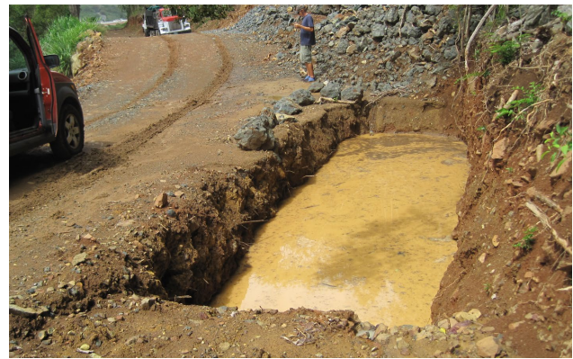
Sediment trap excavated along a construction access road on the east end of St. Thomas.
