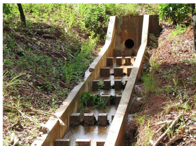
(Top) Outfall with no protection. (Middle) Outfall with some stone and vetiver. Stone should wrap fully around the pipe. (Bottom) Concrete headwall and energy dissipators at outfall location on a slope.
