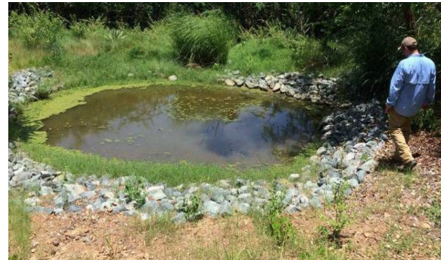
Trap design variant with rock-line side slopes and outlet with vetiver grass on bottom for trapping sediment.
