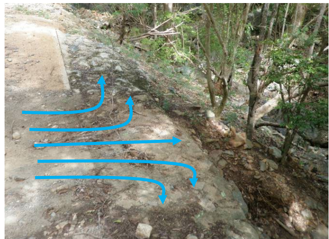
Outlet from dip showing grouted stone level spreader and energy dissipator to slow flows. Remove accumulated sediment, vegetation, and other buildup.
