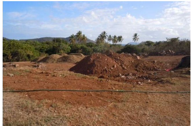
Clear cutting of the entire site at one time eliminates any potential to protect trees or reduce the amount of exposed soil that now requires stabilization.
