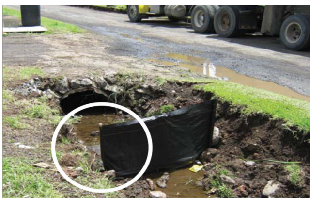
(Top) Check dam needs maintenance. Accumulated sediment should be removed, and the stone adjusted to extend across the full channel width to prevent bypass. (Bottom) Do not use silt fence for check dams. Checks should extend fully across ditch to prevent erosive bypass and have a lower center to allow for controlled spillover.
