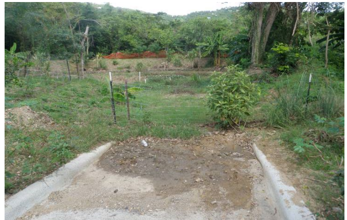
This sediment forebay to a detention pond in Coral Bay will require ongoing maintenance to remove accumulated sediment for the basin to properly function.
