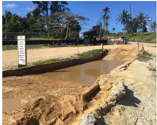
Washing tires of construction vehicles can be a good way to prevent sediment from leaving the site. Tire washes should be designed to manage muddy water.
