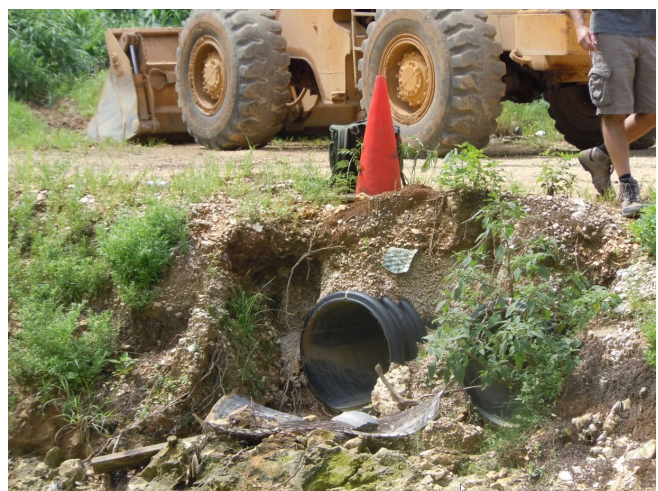
Concentrated flows at the end of a discharge pipe can cause erosion and scour if the outlet is not stabilized or flow velocities are too high.
