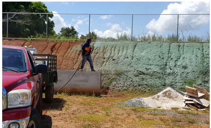
Erosion gullies on an exposed steep slope are being stabilized with vegetation through hydroseeding (photo credit: Protectores de Cuencas).
