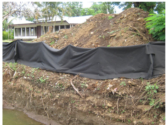
(Top) Properly installed silt fence. (Bottom) Fencing improperly installed—no trenching, incorrect fabric, and too close to the stream/gut.
