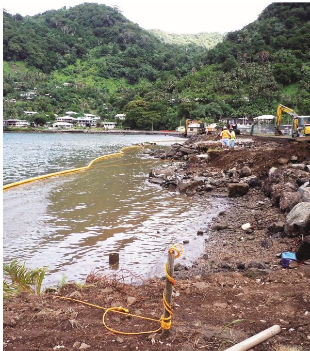
Anchor stakes hold curtain in place. Turbidity curtains are the last line of defense.
