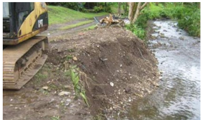
No protection was provided for this stream during adjacent site construction.
