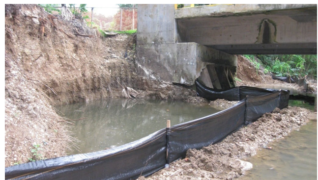
(Top) Examples of cofferdams made from sheet metal and (middle) sandbags (photos from NCDOT), and (middle) inflatable bladder. (Bottom) Silt fence may not be best choice.
