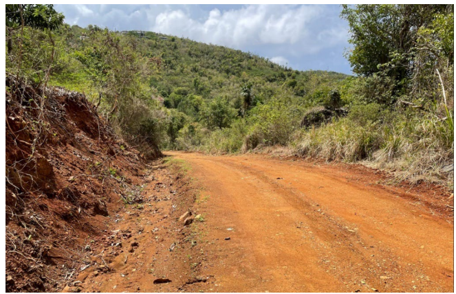
Unpaved roads should not be the source of sediment plumes in the bay. They should be designed for drainage to minimize surface erosion and overall maintenance burden, regardless of temporary or permanent status.
