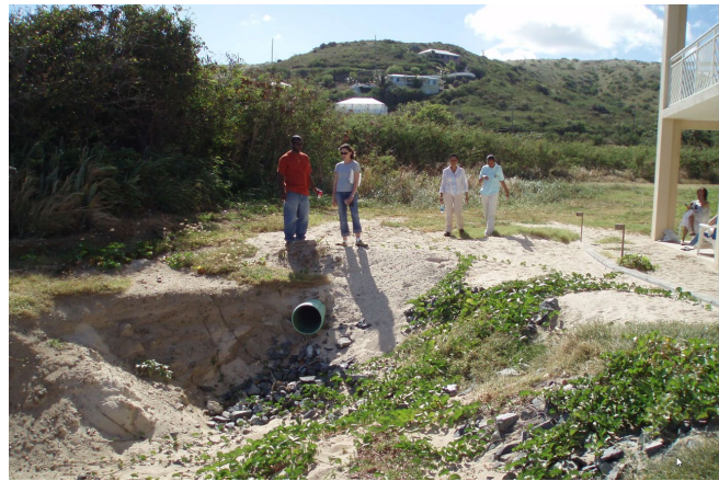
Outfall protection needed at this outlet onto an erodible beach.
