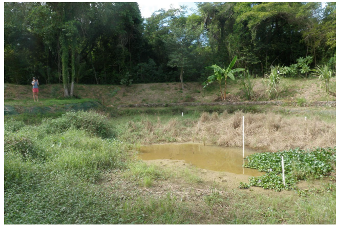
This ponding basin retrofit was installed to manage flooding on Kingshill Rd. in Coral Bay on St. John.
