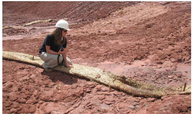
(Top) Compost socks filter fine sediments from runoff (photo: Pacific Unlimited); (Bottom) straw filled wattles do not hold up well and offer minimal filtering benefit.
