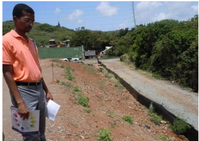
Silt fence is a commonly used perimeter control device to keep sediment from leaving a site.
