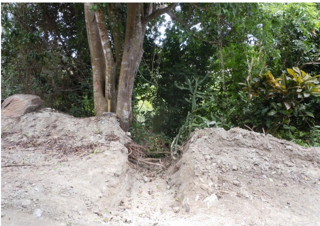
This turnout was added after the fact to address drainage issues on an unpaved access to a residential construction site on St. John. The outlet is not protected, and runoff is not conveyed to a filtering area. This type of ad hoc drainage causes offsite sedimentation and illustrates poor site design and erosion control planning.
