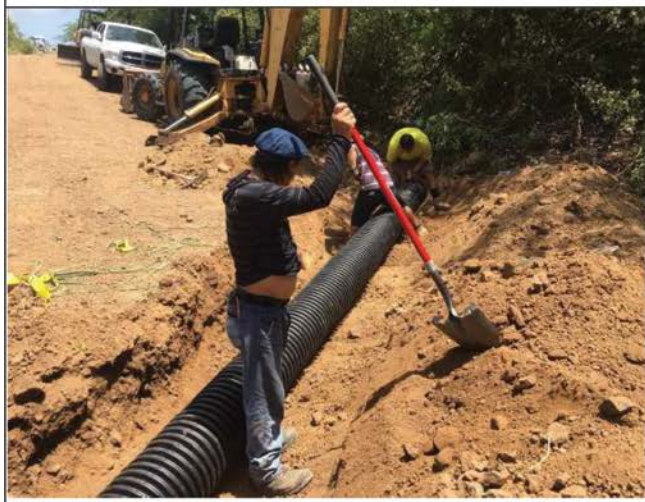
Cross-pipe installation trench should be deep enough to match ditch invert and natural ground level.
