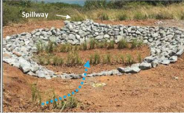
Trap design variant with rock-line side slopes and overflow spillway with vetiver grass on bottom.
