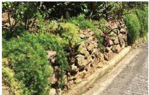
Slope Stabilization: Vegetation, stone, matting, or combination of techniques to prevent erosion of cut or fill slopes.
