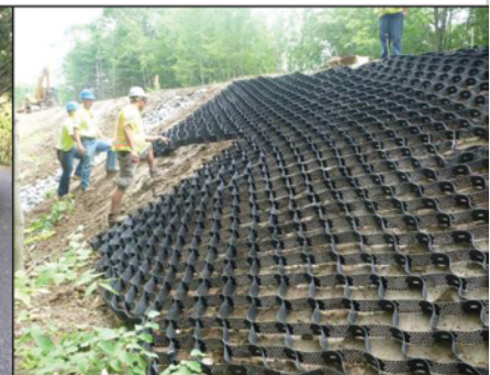
Example of geosynthetic soil containment cells used on road outslope to hold soil in place for subsequent planting.
