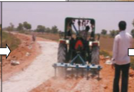
Multiple passes with tractor pulling tiller or disks can be used to mix soil/ aggregate with cement.
