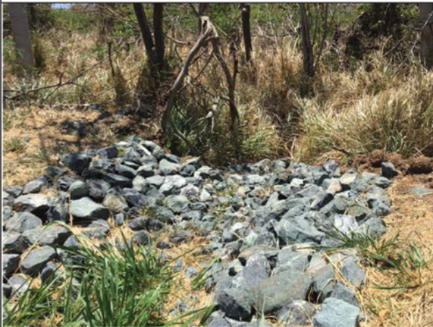
Rock aprons at outlet pipes are good if you have a level area where flow can be dissipated into a vegetated buffer.
