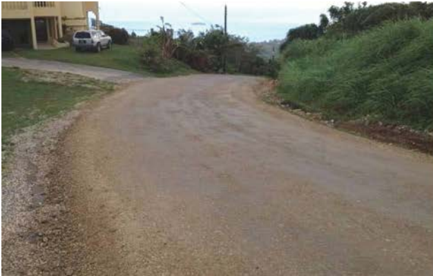
Soil/Aggregate Stabilizers: Additive used to increase adhesion and longevity of road base materials. Some products may be toxic to aquatic life and are not recommended for use in sensitive watersheds.
