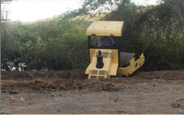
Proper compaction of dam/outlet berm with roller or hand held compactor is a critical step in construction.
