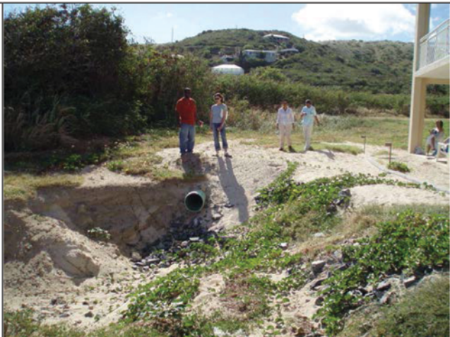
Outlets without stabilization can lead to erosion and headcutting.
