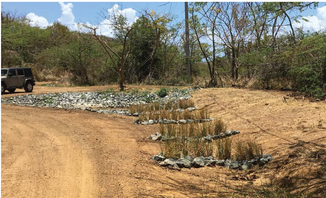
Example of recently planted vetiver-rock check dams leading to a sediment trap on Culebra, Puerto Rico.
