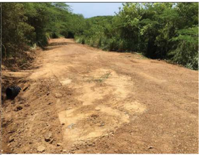
Consider adding compacted fill on top to provide sufficient cover. This could become a grade break.
