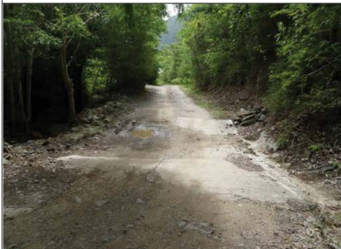
Dip intersects ditch (left side of photo) and discharges downslope (on the right). If not pitched enough or if outlet blocked by vegetation, dip can fill with sediment.
