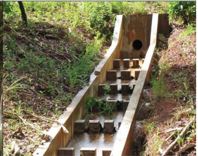
Probably overkill for short road segment outlets, but more formal energy dissipation for higher volume flows is an option.
