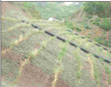
Rows of vetiver grass recently planted along road outslope. Hydroseeding is visible between rows to help hold exposed soil in place while vetiver establishes.
