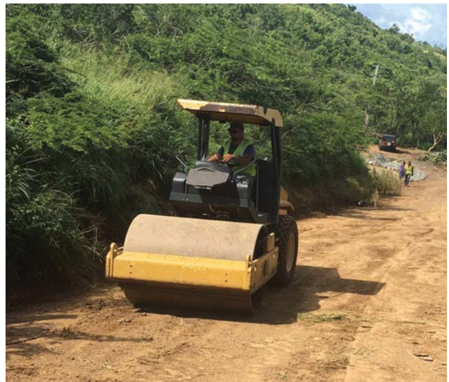
Ensuring proper compaction of the road surface is critical to extending the life of the road surface.
