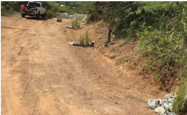
Ditch: parabolic, V-cut, or trapezoidal channel adjacent to road used to convey concentrated flows; usually has check dams and is vegetated or stone lined.
