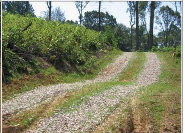
Rock reinforced broad-based dips are easily traversed by cars. Notice no ditch interception here, so concrete not necessary.
