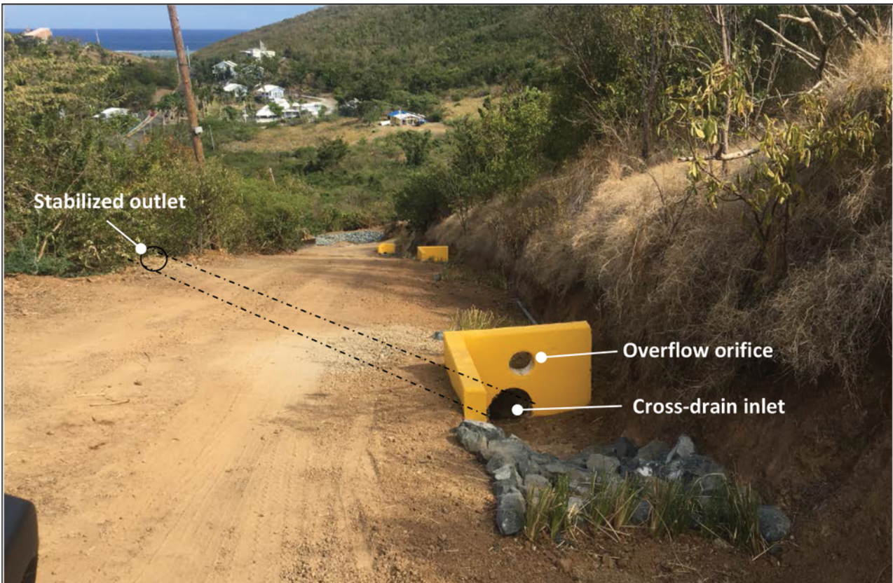
Use of headwalls for cross-drains on Culebra, Puerto Rico to increase visibility and stability around pipe inlets. The headwall helps to funnel flow into pipe. An overflow orifice is provided in case inlet becomes clogged.
