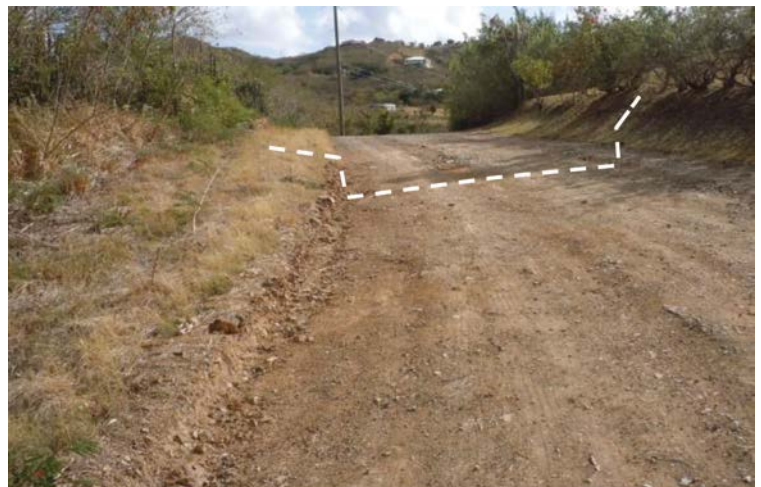
Once a road becomes entrenched, it becomes a conduit for water. If drainage alternatives such as ditching and turnouts are impractical, the road profile will need to be raised.
