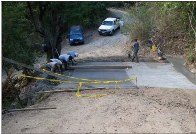
Construction of concrete dip in two pours to allow vehicular access during construction.
