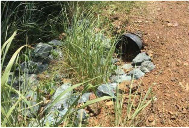
Stabilized Outfall: stone, vegetation, or other method of preventing scour at outlet structures.
