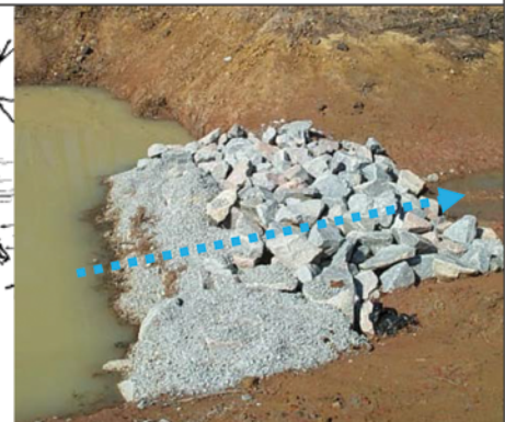
Create a filter using smaller sized rock on the inside of rock dams.
