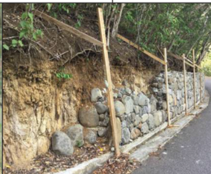
Example of a stone revetment used to stabilize road banks. Gabion baskets are also popular. Consider options that combine both rock with native vegetation.
