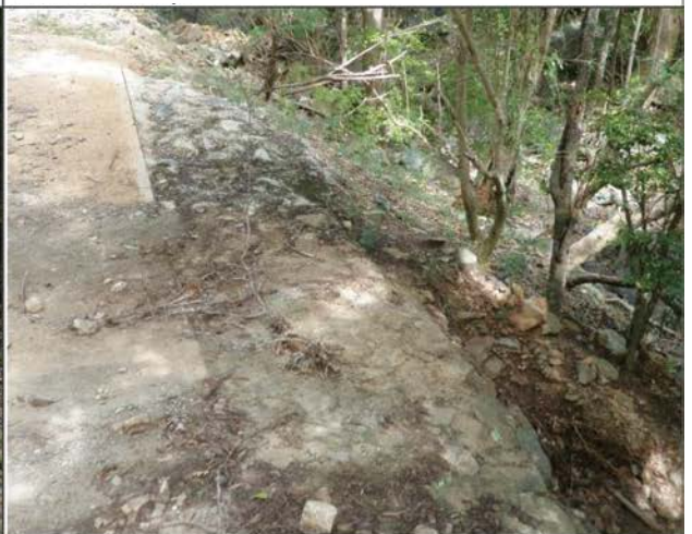
Outlet should be stabilized and include a level spreader (as shown here) or energy dissipator to slow and spread discharged flows.
