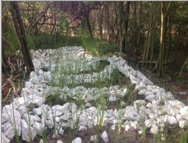
Design variant of a rock channel outlet using combination of rock and vetiver rows to dissipate flows.
