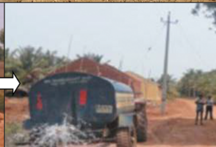
Use of a water truck to wet mixture before final grading and compaction.
