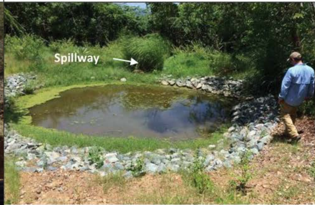
Traps can become permanent drainage control features that provide water quality treatment prior to discharge.
