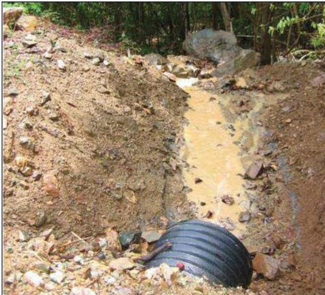
Lack of outlet protection at this newly installed cross-drain leads to erosion of slope at pipe exit.
