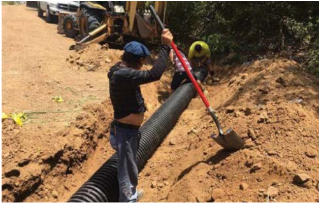
Cross-drain: piped or open top culvert that conveys concentrated flows from one side of road to other, usually from an inside ditch to the outslope.
