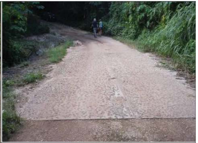
Stones embedded in concrete low-water crossing to improve vehicle traction during wet weather.
