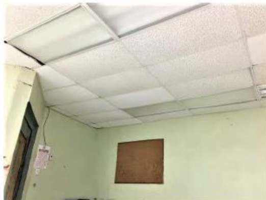
Typical sagging acoustical ceiling tile (ACT) and metal grid
