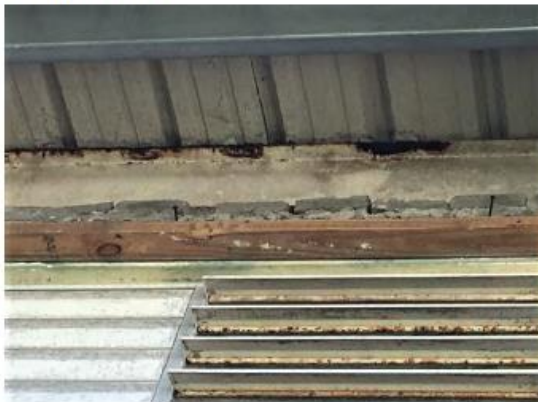
Damaged concrete wall above window below soffit
