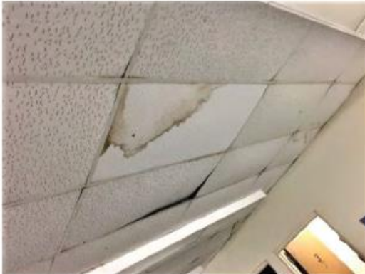
Sagging/stained acoustical ceiling tiles (ACT) & grid
