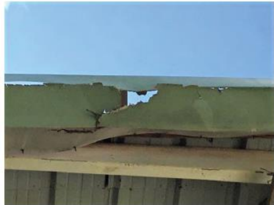
Damaged custom-made aluminum gutter & flashing
