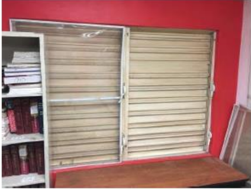
Damaged window screens
