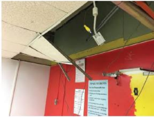
Damaged ACT metal grid
