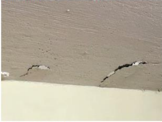
Spall on concrete ceiling
