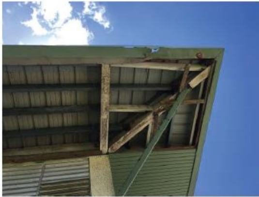
Damaged soffit NE
