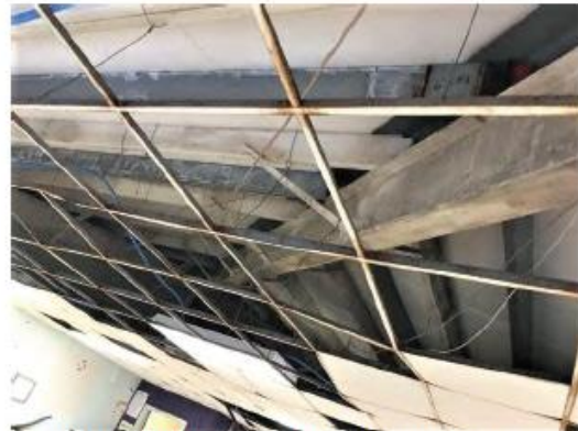
Damaged acoustical ceiling tiles (AC) metal grid
