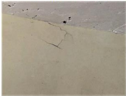
Spall on concrete wall
