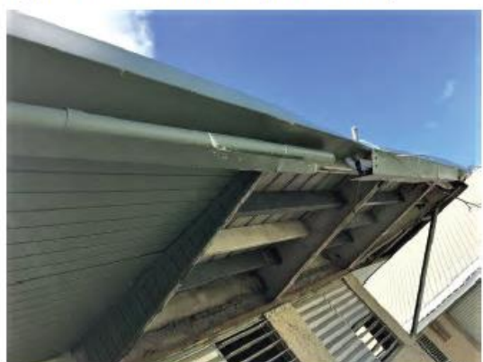
Damaged soffit, aluminum gutter, PVC storm water pipe
