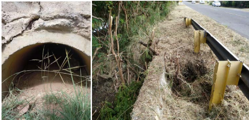
Figure 8. Blocked Culvert (Seven Flags) and Undermining of Culvert Headwall (Southgate East Gut)
