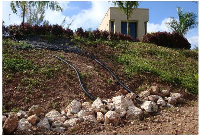
Example of a pipe slope drain used to temporarily convey driveway runoff to stone apron below unvegetated slope.
