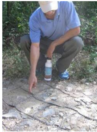
Checking Geoweb installation on St. John to evaluate surface compaction and material loss over time.
