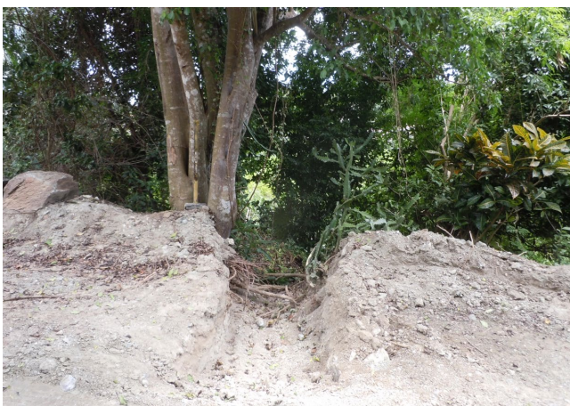
This turnout was added after the fact to address drainage issues on an unpaved access to a residential construction site on St. John. The outlet is not protected, and runoff is not conveyed to a filtering area. This type of ad hoc drainage causes offsite sedimentation and illustrates poor site design and erosion control planning.
