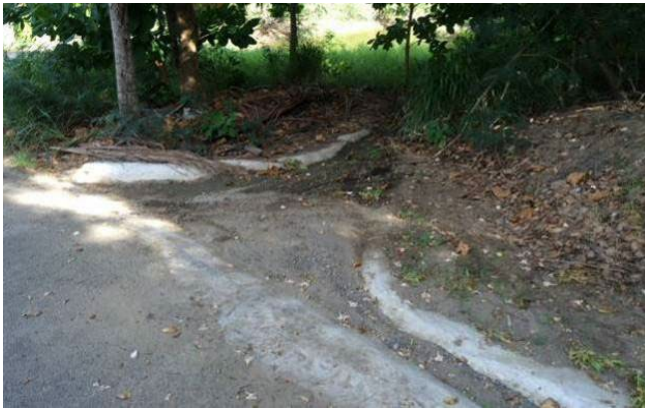
This concrete turnout directs runoff from an unpaved road to a stormwater ponding basin. Sediment deposited in the turnout needs to be removed to ensure continued drainage. Maintenance can easily be conducted with a shovel.
