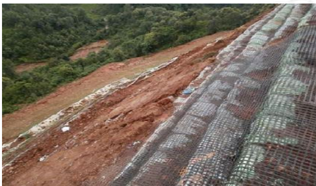
Figure 4.15 Geogrids layers stacked with fill to stabilize a slope (detail from VT Better Backroads Manual).
