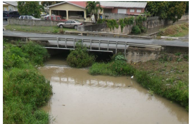
Structural practices will need to be sized to attenuate peak discharge rates to minimize downstream flooding (photo credit: Frank Galdo).
