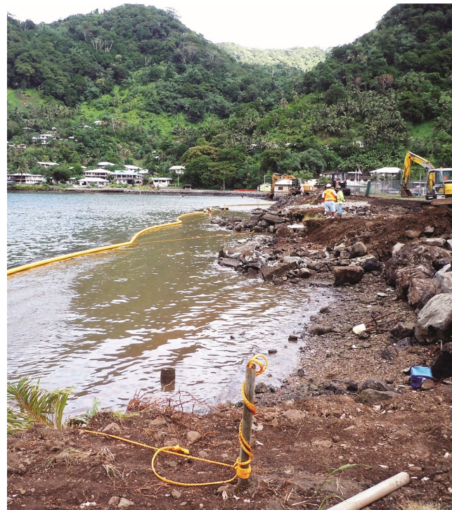
Anchor stakes hold curtain in place. Turbidity curtains are the last line of defense.
