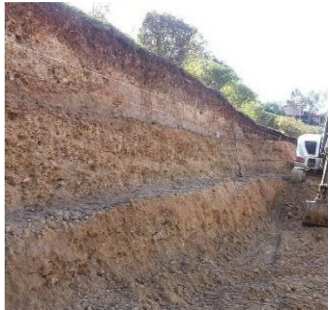
Cutting benches into an almost vertical slope to help support walls and plantings.
