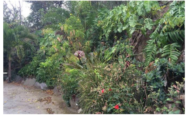
This cut slope on a residential driveway in the BVI was stabilized with stone walls and landscape vegetation—a win/win for the homeowner and downstream coral reefs!
