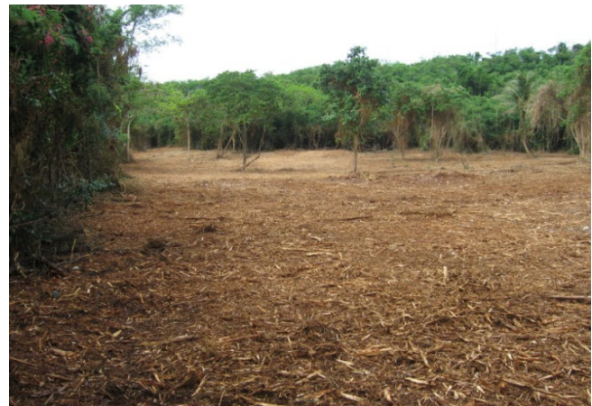
Mulching on site as clearing occurs is standard practice; however, clearing only the area needed for construction (site fingerprinting) and leaving as much natural vegetation in place as possible, is the preferred approach.
