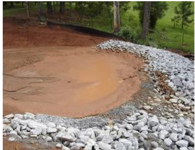
Remove accumulated sediment when trap capacity is less than 1/2 the design volume to avoid a situation where there is not enough storage capacity for the next storm event.
