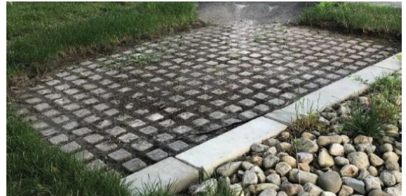
Examples of hardened sediment forebays (with permeable pavers) for easy maintenance that will also drain down after storms.
