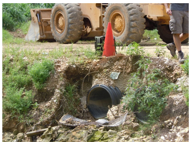
Concentrated flows at the end of a discharge pipe can cause erosion and scour if the outlet is not stabilized or flow velocities are too high.
