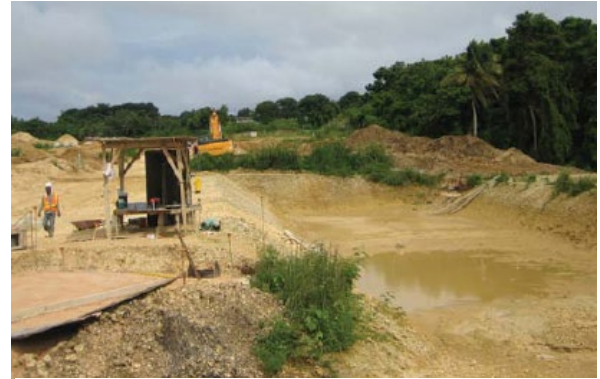
Examples of sediment basins (bottom photo: Guam EPA)
