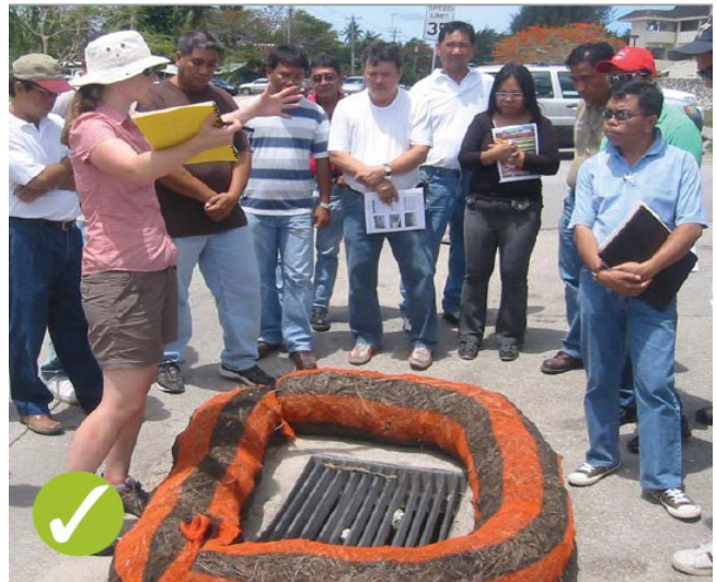
(TOP) Good example of a filter sock inlet protection used on pavement that filters sediment while still allowing drainage.
