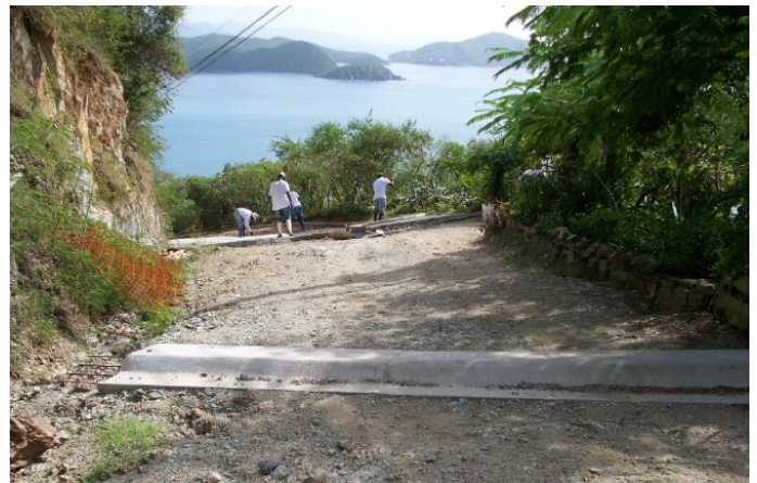
Unpaved roads on steep, highly erodible slopes are one of the most significant sources of sediment to nearshore waters in the USVI. Strategic paving and use of appropriate drainage practices can have a direct impact on the quality of water resources (photo: Coral Bay Community Council).
