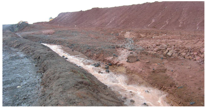
Moving runoff through the site without causing erosion can be a challenge. Limiting drainage area contributions, stabilizing flow paths and slowing velocities are key strategies.
