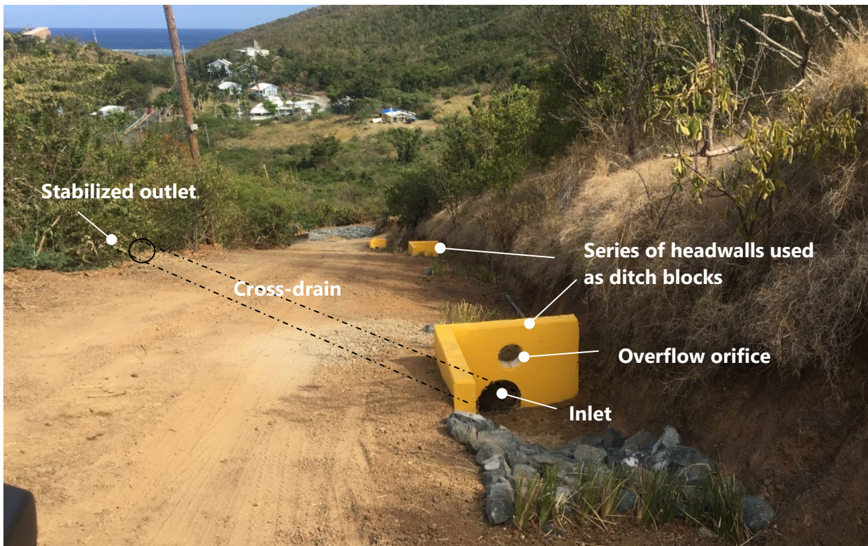
Cross-drains were used to replace water bars along this demonstration road segment. Headwalls with overflow orifice were added with energy dissipators (rock and vetiver grass) in the ditch. The key to success with this installation is rapid stabilization of the ditch and prevention of headwall run-around.
