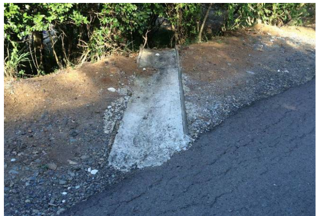
Concrete turnout from a recently paved road takes runoff down to a vegetated filter strip.
