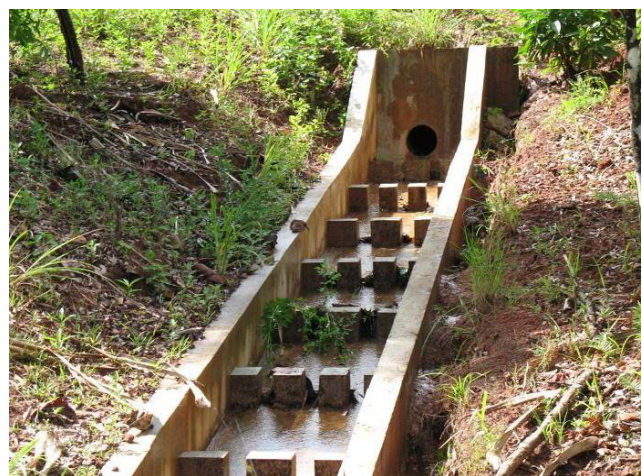
(Top) Outfall with no protection. (Middle) Outfall with some stone and vetiver. Stone should wrap fully around the pipe. (Bottom) Concrete headwall and energy dissipators at outfall location on a slope.
