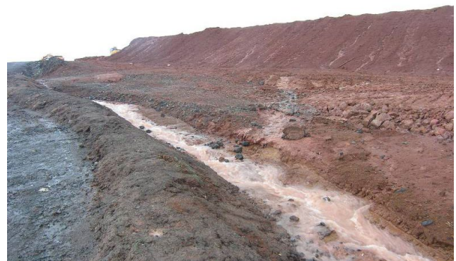
This ditch is carrying high velocity runoff through an exposed construction site. The channel should be stabilized and have check dams to slow runoff and prevent erosion.
