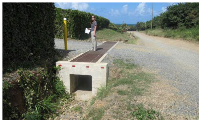
Concrete culvert with metal trench grate carries ditch flow and collects surface drainage from unpaved drive on Seven Flags Rd. in St. Croix.
