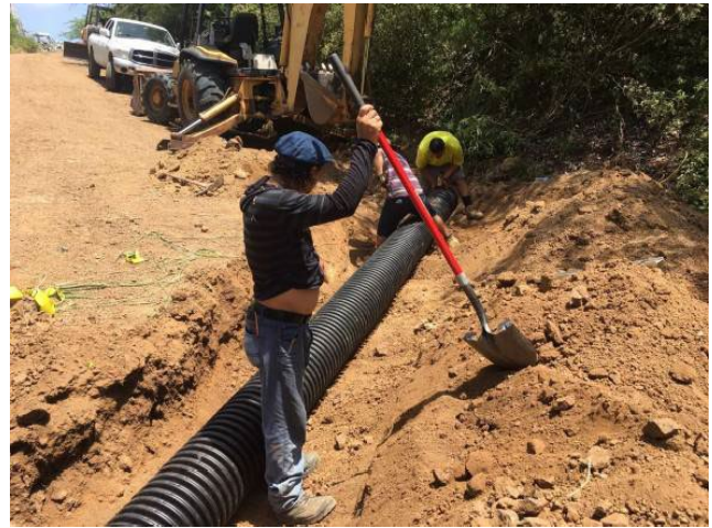
Digging trench for cross drain installation on Culebra, PR. Notice the pipe is laid at a 30–45-degree angle to road to better intercept ditch.
