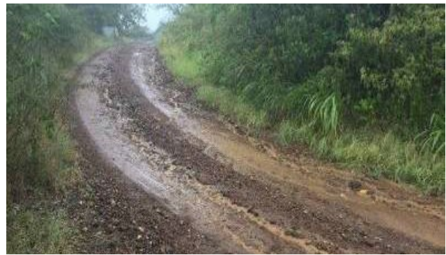
The last place you want concentrated flows is in the travel lane since this will lead to erosion.
