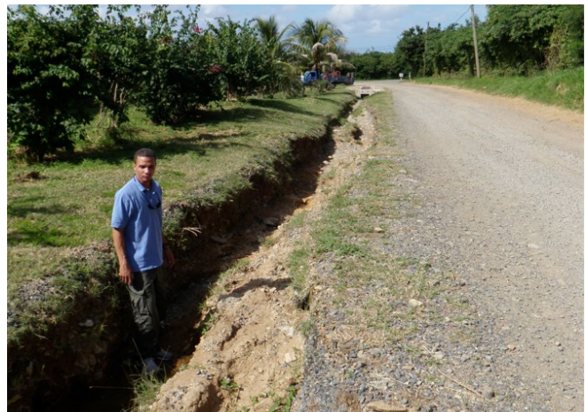
High volumes and velocities can lead to ditch erosion and backup at undersized driveway culverts.
