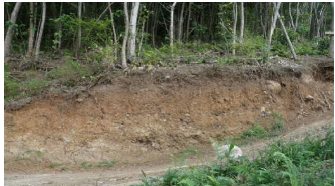
Vertical cut slope along the inside of an unpaved road.
