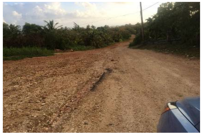
Excessive road widths can create a much larger disturbance footprint than needed, lead to increased erosion and sediment loading, and require more extensive maintenance than originally planned.
