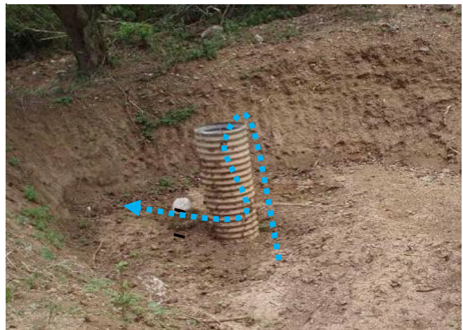
Vertical standpipe – should be perforated, wrapped with geotextile fabric or a rock filter.
