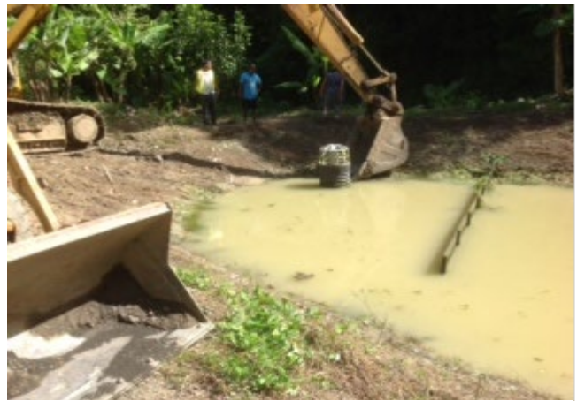
Excavation of accumulated sediment during maintenance of sediment basin. Note outlet pipe with trash rack and baffle.
