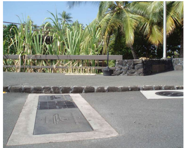
Use of underground proprietary device prior to bioretention on the Big Island of Hawaii.
