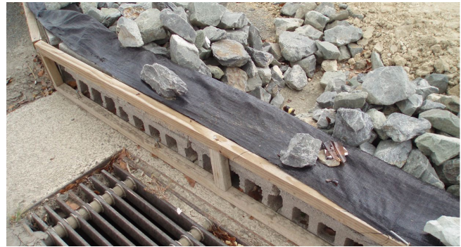
Inlet and outlet protection is as much an art as it is a science. You may have to be creative with accessible materials.
