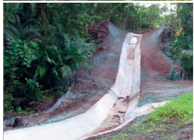
Examples lined waterways: (Top) erosion control matting; (middle) stone and grass; and (Bottom) concrete-lined waterway on a steep slope.
