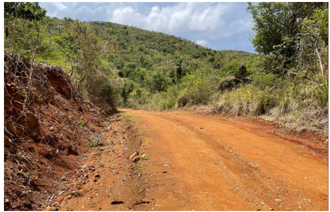
Unpaved roads should not be the source of sediment plumes in the bay. They should be designed for drainage to minimize surface erosion and overall maintenance burden, regardless of temporary or permanent status.
