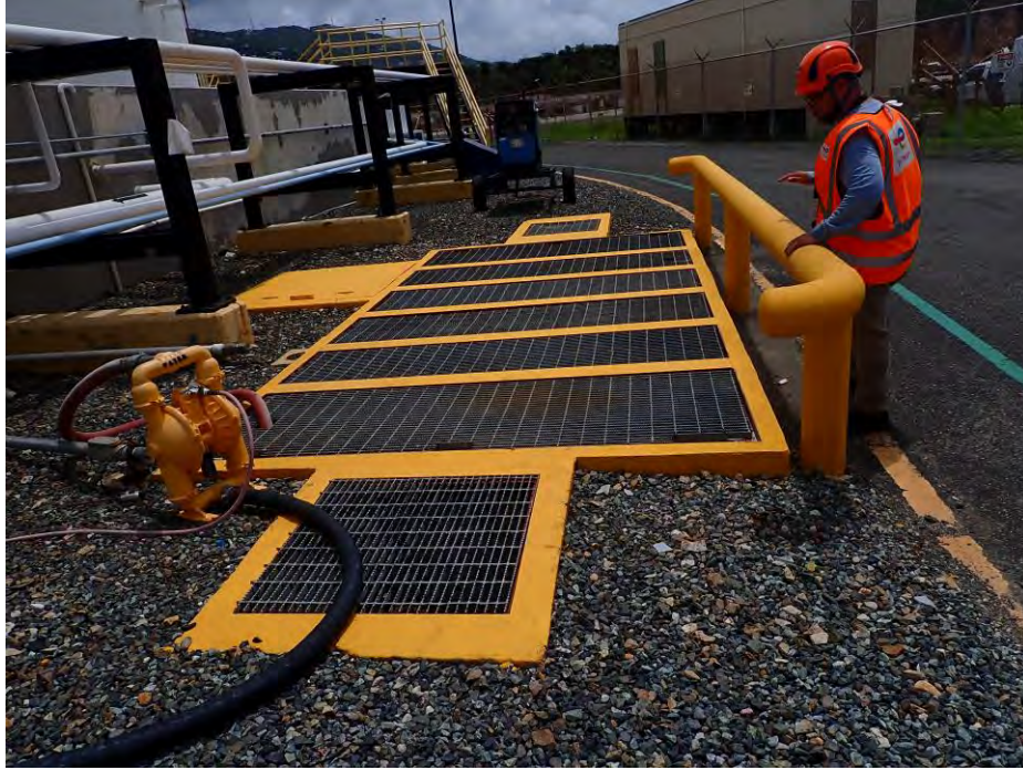
Figure 5.02.06.01 The grated, underground three chambered storm water basin acts by separating clean water from fuel via density separation. Water that falls into containment areas is pumped into the water/fuel separator and only clean water is released.
