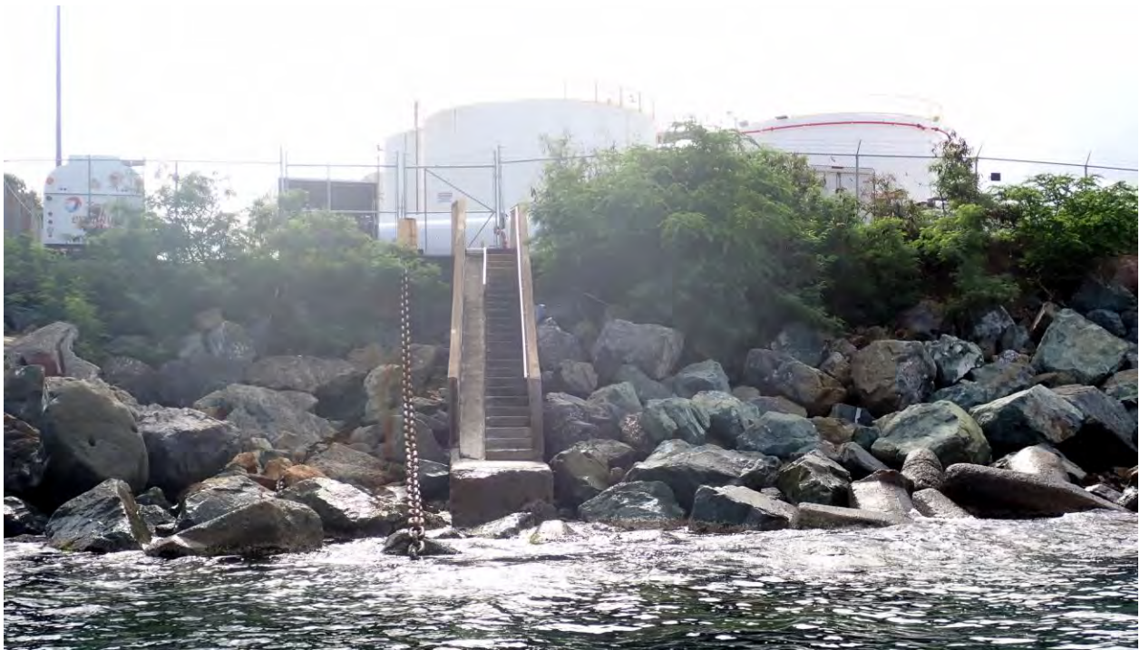
Figure 5.02.03.08 The TotalEnergies Terminal steel pipeline is encased in concrete and descends down the shoreline covered in large boulders on the west side of the property to the sea floor.
