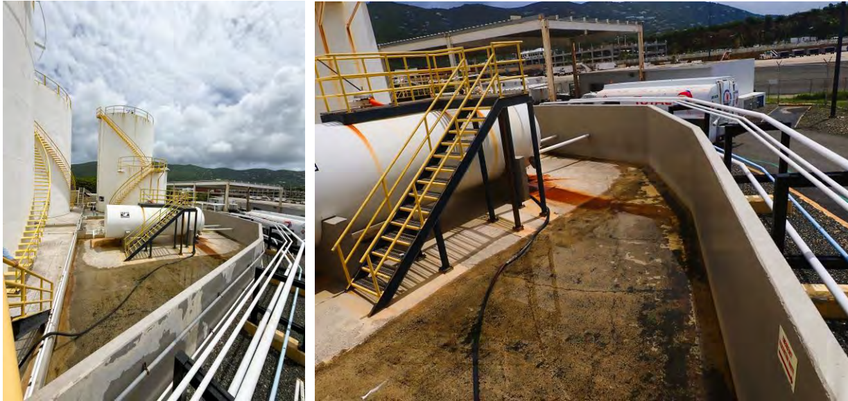
Figure 5.02.03.02 The tanks are surrounded by a 9' concrete retaining wall as required by 40 CFR Part 112 which stipulates that a secondary containment for bulk storage containers must hold 110% of the container volume.
