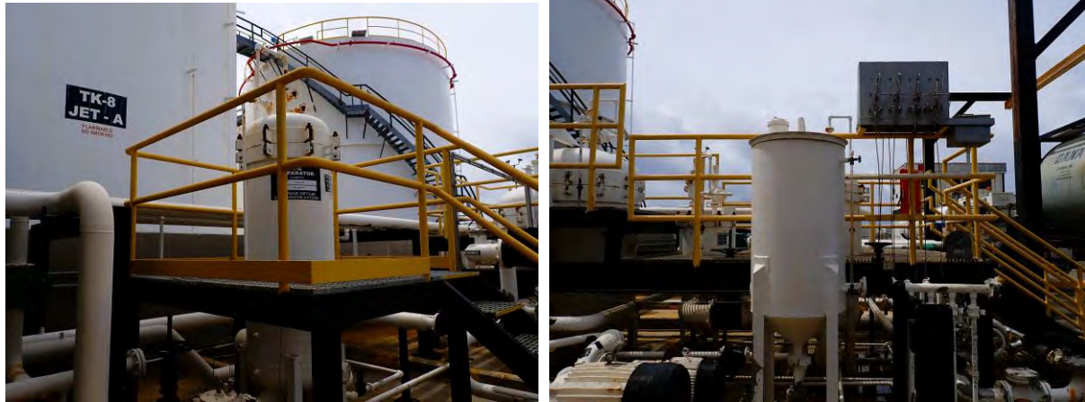
Figure 5.02.03.04 A double filtration system is used inline when transferring Jet Fuel from storage tanks to the filling tank. This manifold/filtration area is on the west side of the storage tanks near the filling station.
