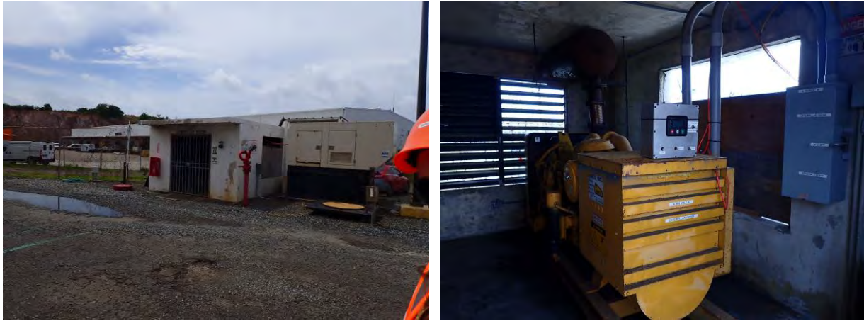
Figure 5.02.03.11 A small concrete building housing a 150 KW generator sits on the southern edge of the property. An additional out of service 100 KW generator is located outside of the structure. Improvements included relocating generators and installing electrical cabinets for power distribution in the protected concrete building.
