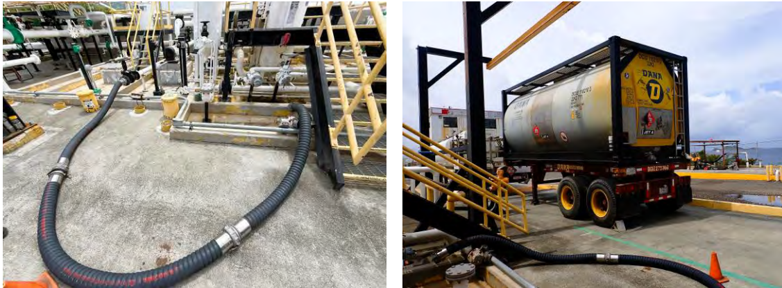
Figure 5.02.3.05 The diesel truck filling area is adjacent to the manifold and filtration area
