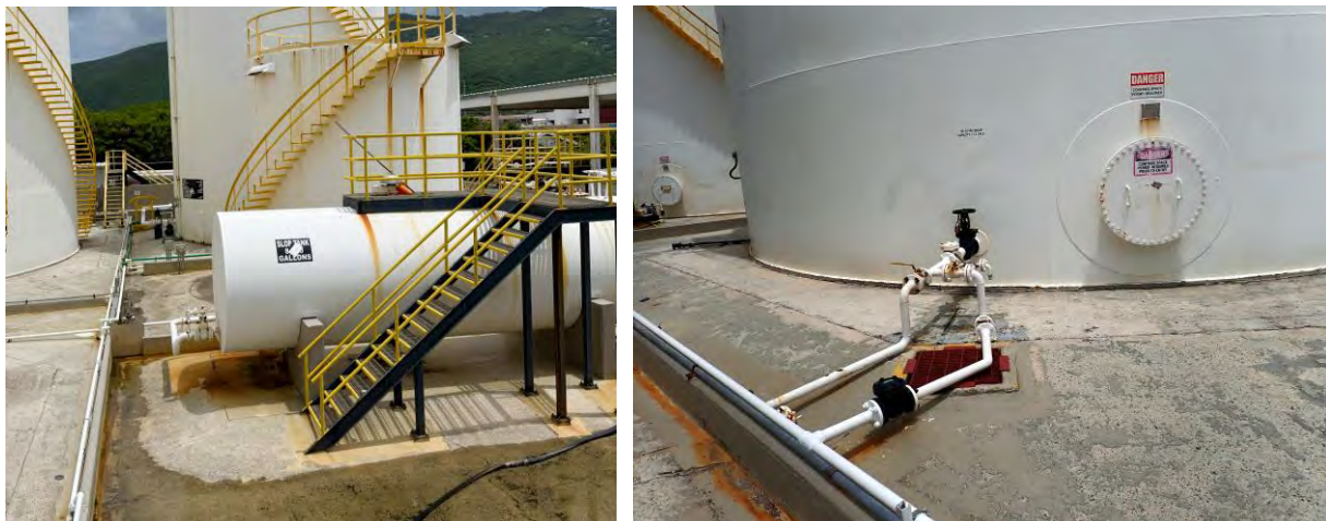
Figure 5.02.03.03 Fuel is sampled daily from the bottom of the tanks for roof leakage or internal condensation; any water collected is piped to the slop tank where it is stored until removal by an outside contractor.
